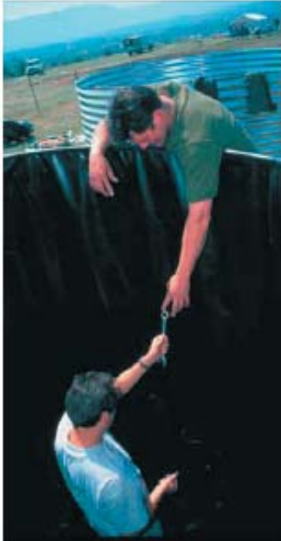
Setting up a water tank at a camp for Kosovan refugees in Macedonia Photo: Howard Davies
