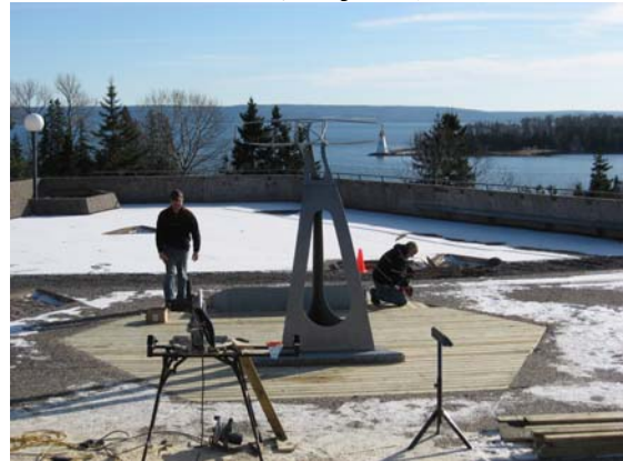
Deryck Chapman and Gary Pierrard put the finishing touches on the new decking around the Silver Dart monument.
